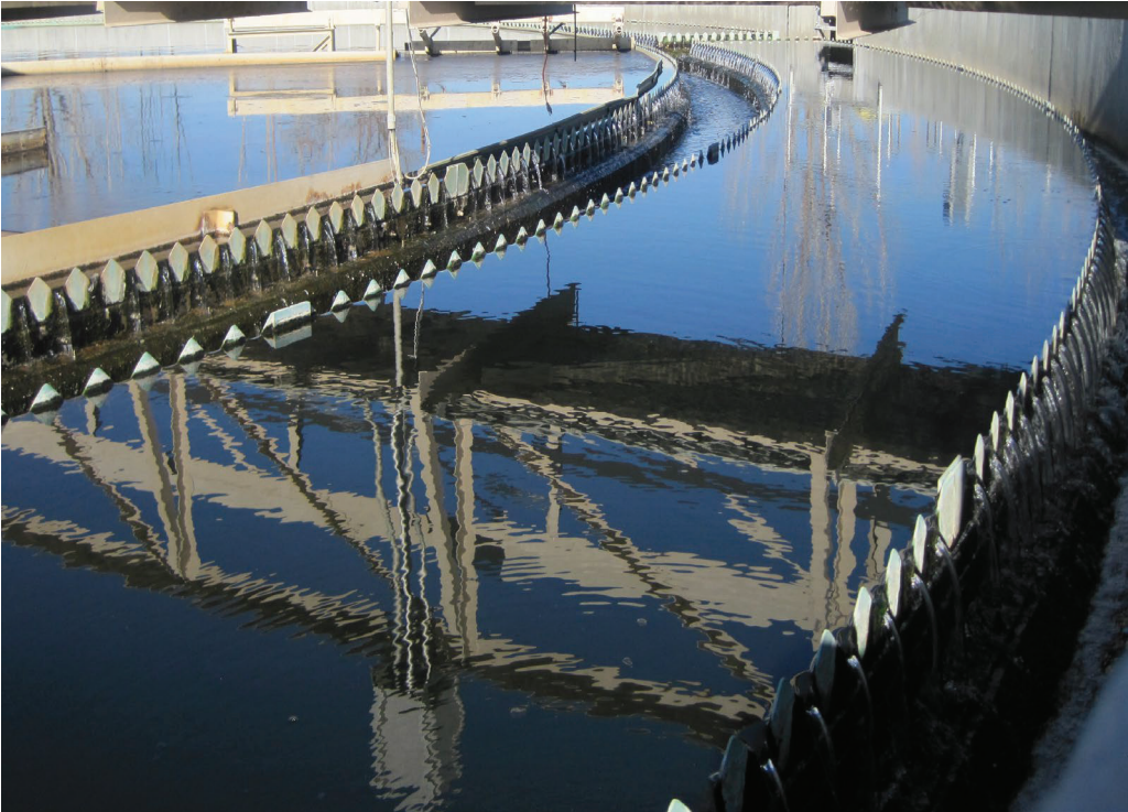
Southside Water Reclamation Plant (SWRP) Skimmer Reflection
