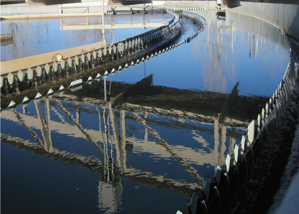
Southside Water Reclamation Plant (SWRP) Skimmer Reflection
