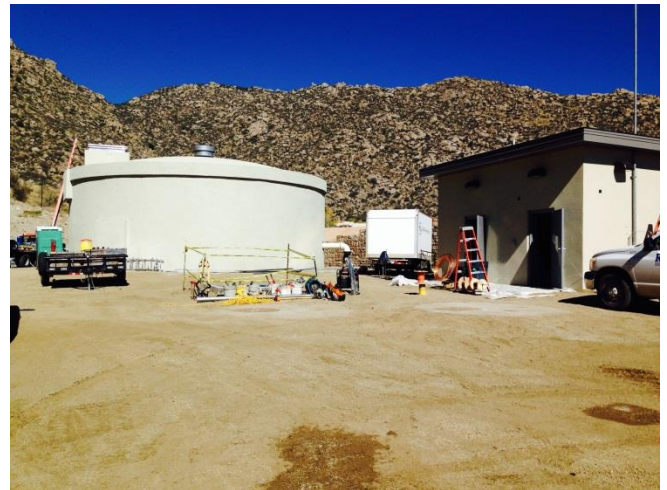
(Above) Photo of reservoir and chlorination building under construction in Echo Canyon (October 2014).
